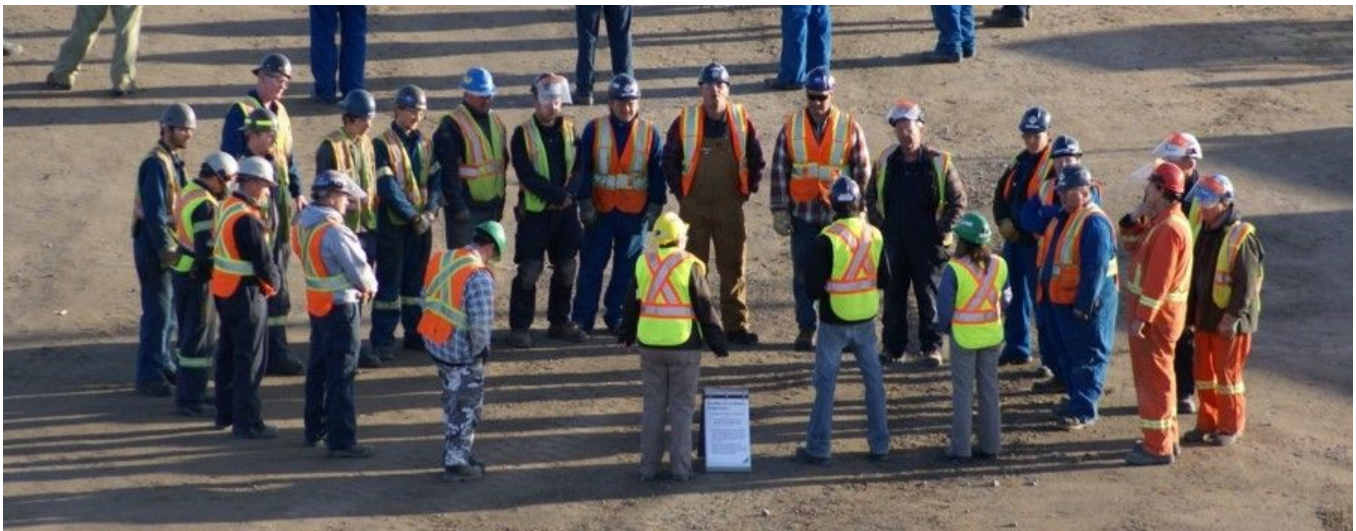
Regular toolbox meetings to review the work hazards and requirements across all trades is a good practice.
