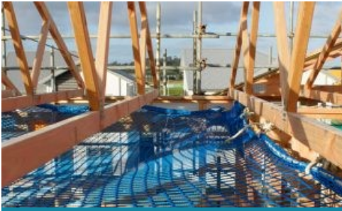
Safety net securely installed under trusses
