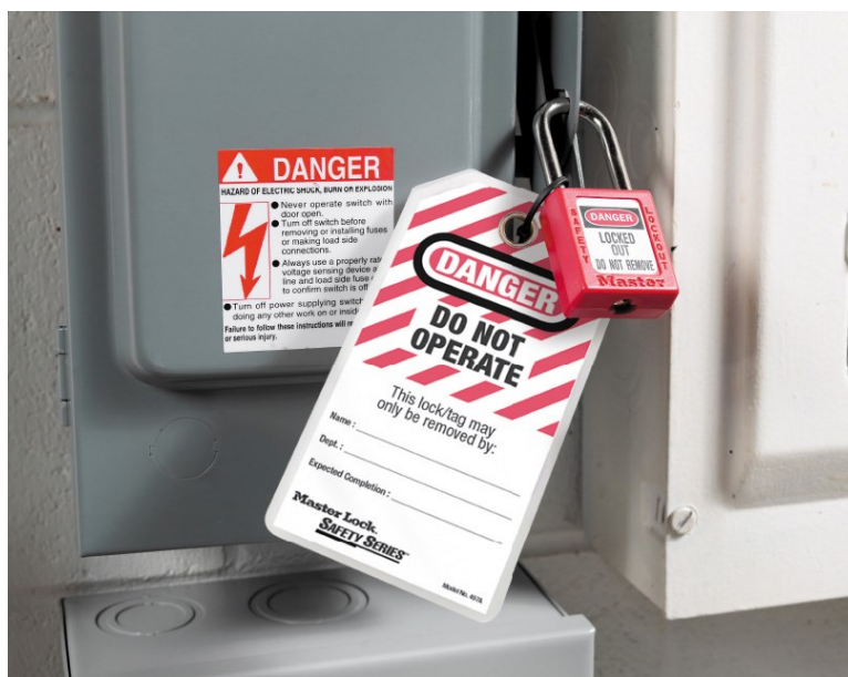
Figure 3. Example of proper Lock-out Tag-out
