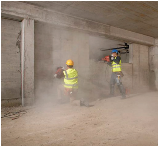
Figure 2—Silica dust exposure after 3 minutes of drilling.
